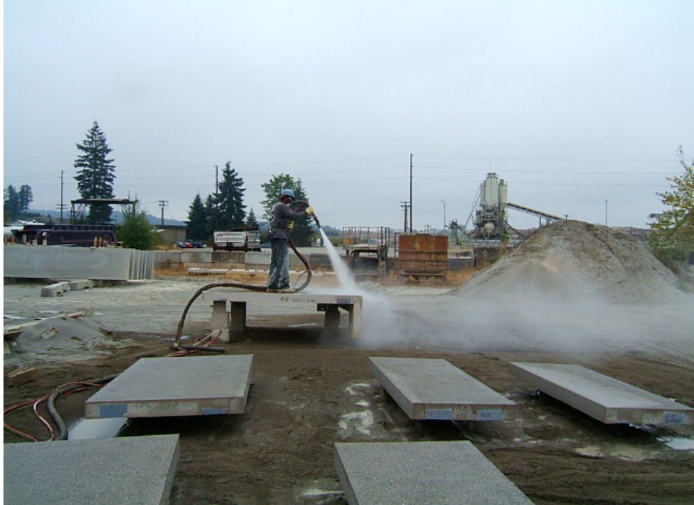
Figure 6. At the large station, building panels are placed on blocks about 1 to 2 feet above the ground. The worker stands on the ground or on the object to perform abrasive blasting. At regular intervals, the worker rinses off the object with water to determine whether the correct finish is being obtained. During the study, the worker was exposing some of the underlying aggregate. Note that this wet abrasive blasting process inevitably generates mud and water puddles as depicted. However, the process and work practices suppress the resuspension of dry sand.
