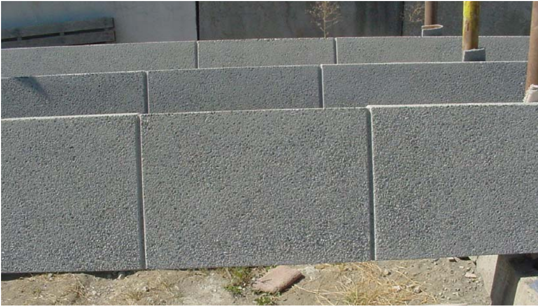
Figure 7. Exposed aggregate after blasting building panels at the large station. The underlying aggregate is clearly visible and the surface appears to have been roughened.
