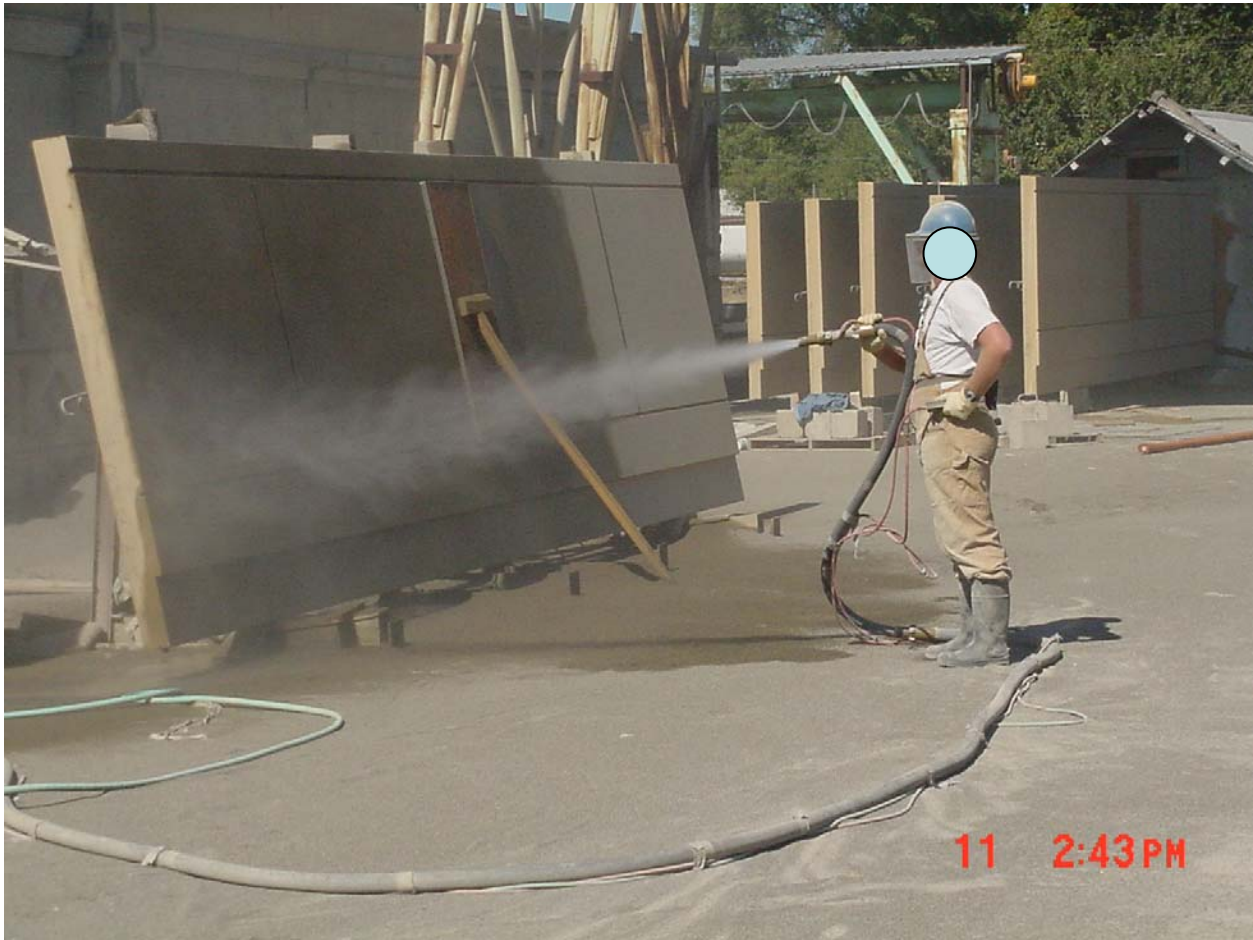
Figure 9. A worker performs wet abrasive blasting on a wall panel at the Crane Way station. The goal was to obtain a uniform color, and only a minimal amount of material was removed. The object thickness was not appreciably reduced. Note that the water drains from the product and the used sand is kept wet.
