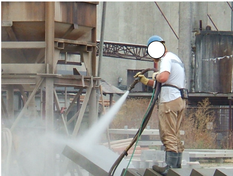
Figure 8. At the small station, the worker performs wet abrasive blasting on fire exit stairs. The bin for filling the abrasive blasting pot is in the background on the left. The aggregate is barely visible.
