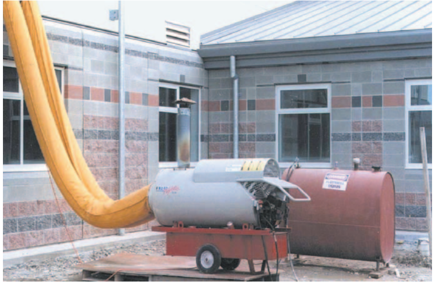
This oil-fueled indirect-fired heater vents emissions outdoors while heated air (free of emissions) is ducted indoors.
