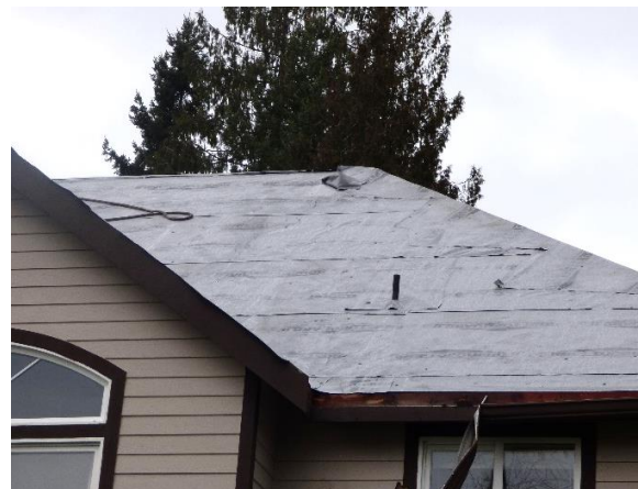
Location where the roofer fell.
